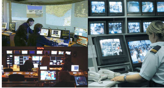
Fig. 2. Various control rooms.
