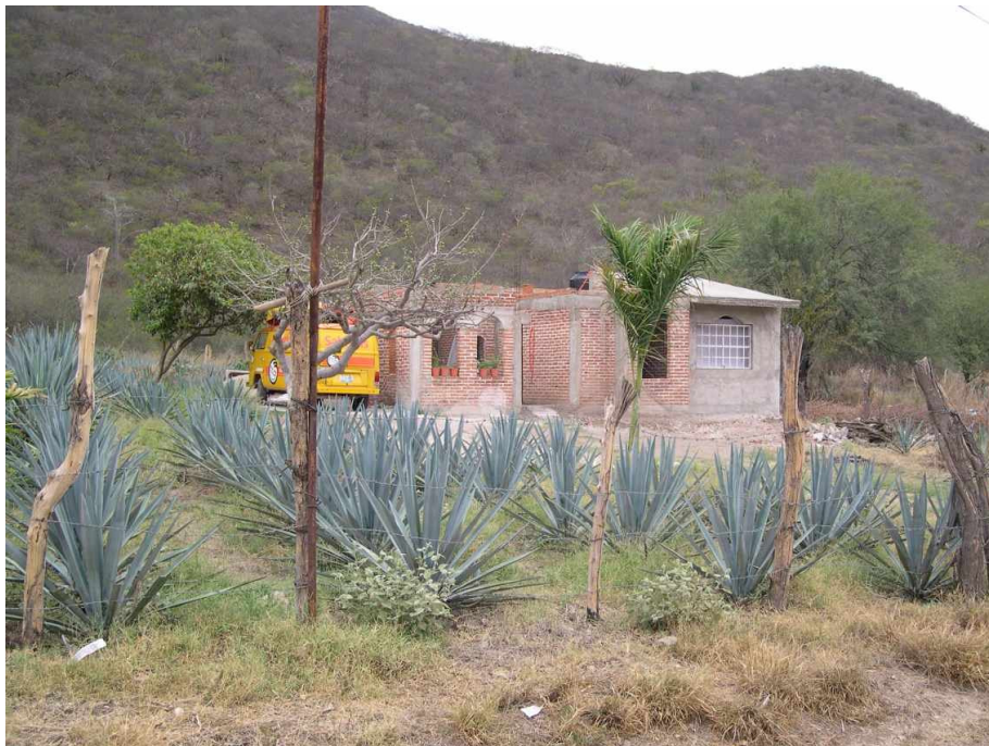
An example of the many houses that are being constructed in Mezquitán. Photo by author (April 2004).
