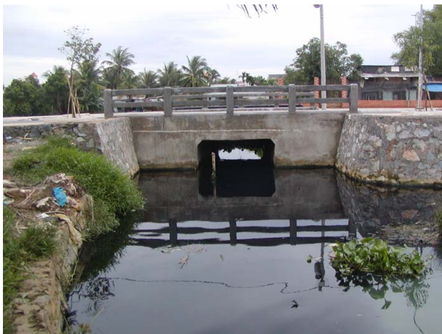
Fig. 6.1 The sewer mouth for run-off from BienHoa Airforce Base in BienHung Lake
