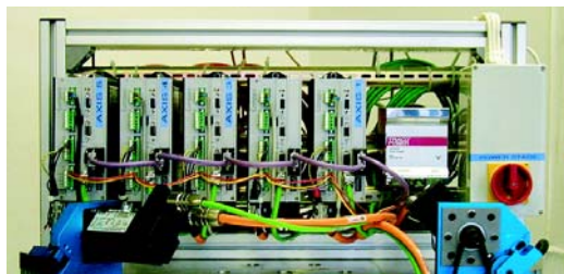
Figure 5: The Control Hardware. The figure shows the 5 drives of our prototype. They contain the PROFIBUS-interface, the control-”intelligence” and the amplifiers.
