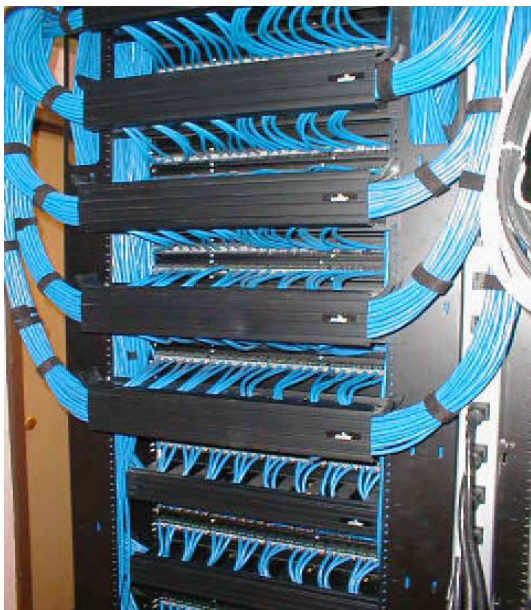
Fig. 13. Two cable rooms, part of the network of the School of Electrical and Computer Engineering at Cornell. Top: one where the old cabling has not been replaced yet; bottom: new infrastructure. The rewiring of our network started around 11/2001, and it is expected that by 4/2002 it will be complete.
