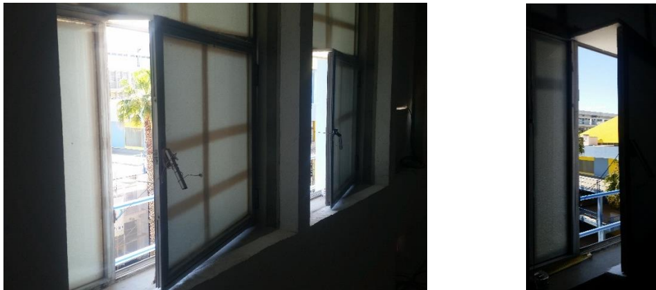
Picture 1 – Example of the two openable windows in BR (left); Example of openable window in SR (right)
