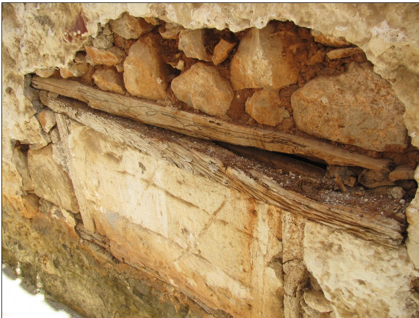
Figure A.69 A premodern house at Korphos made of rubble and locally-derived mortar.
