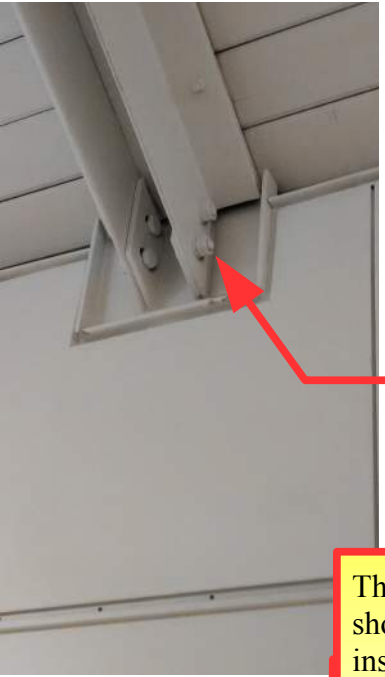
This is one of the identified leak areas. Note metal adjacent to leak.
