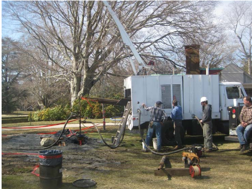
Figure 13: Setting up for hydro-fracturing. Truck is fitted out with a crane and pumps/compressor
