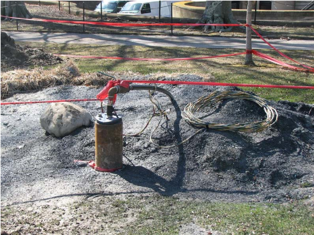
Figure 18: 48-hour drawdown pump test in operation. Pumped water was discharged into drains in the maintenance drive.
