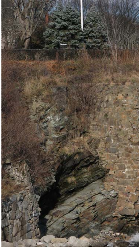
Figure 3: An old well head (at arrow), probably hand-pumped, is found abutting The Breakers on Cliff Walk. Different layers and rock can be seen on the cliffside: overburden, schist, conglomerate, and slate. The schist layer is very wet.
