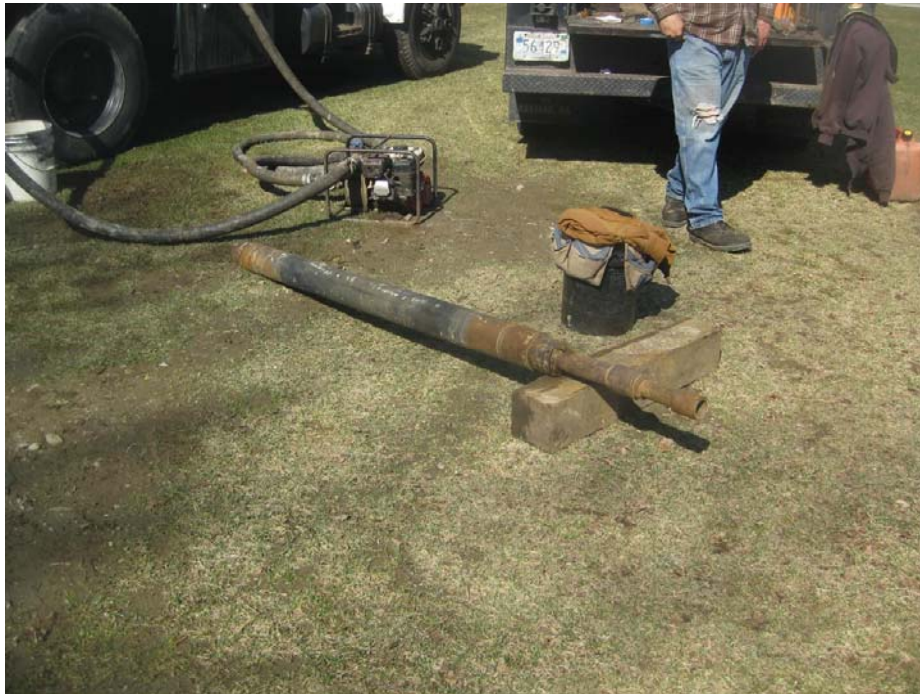
Figure 15: An expandable plug (“packer”) is inflated in the hole at each fracture zone to seal it while compressed air and water is injected through the pipe.
