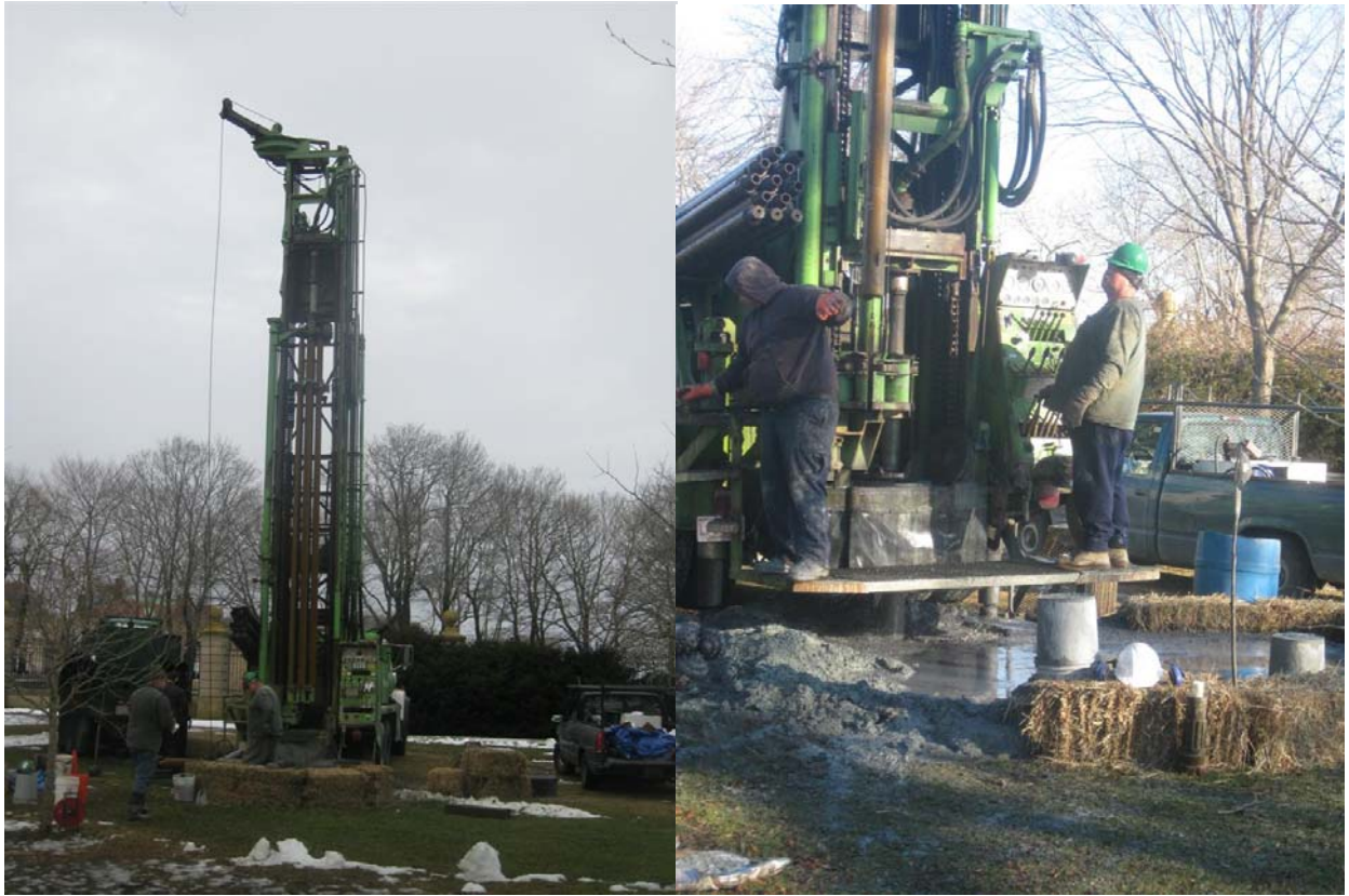
Figure 10: Drilling underway at Drill Target #1. Note hay bales to contain drill slurry. Eventually, a containment pit had to be dug.
