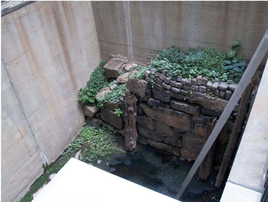
Original Medical College Wood Pilings in an HVAC access area on the Massachusetts General Hospital campus.
