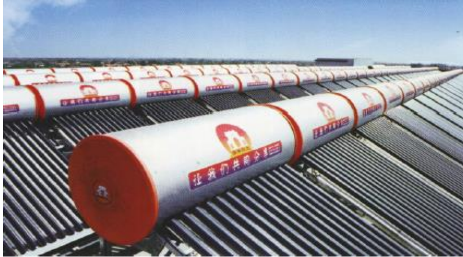
Figure 12. SWH system installed on a rooftop (Li. et al, 2007)
