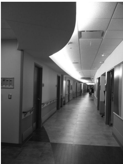
Figure 5.19: Hand Railing Installed in a Slightly Curved Corridor
