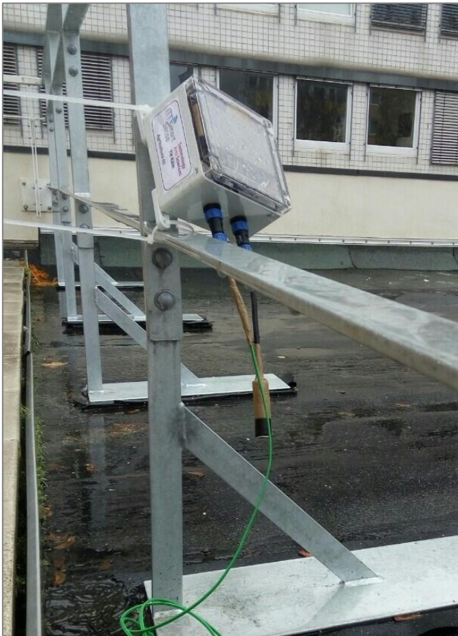
Figure 35: ITT Smart Sense Box installed at ITT's Kalk office
