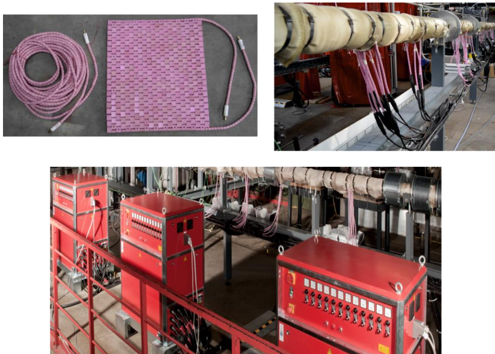
Fig. 16 Heating mat (top left), its arrangement on the pipe surface (top right), and the powering heat treatment units (bottom)
