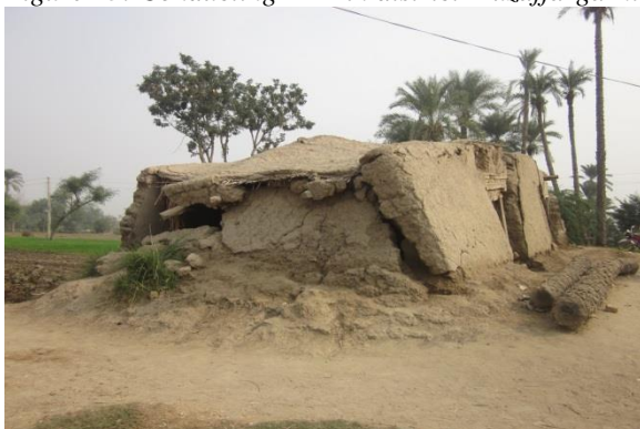
Figure 47: Mud house destroyed by flood.
