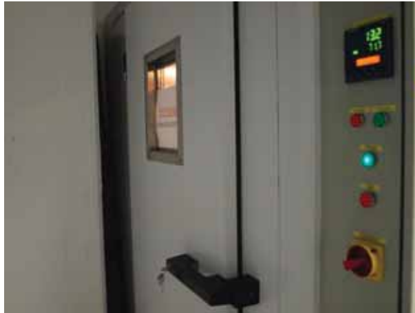
Figure 1: Control panel of the climatic chamber.
