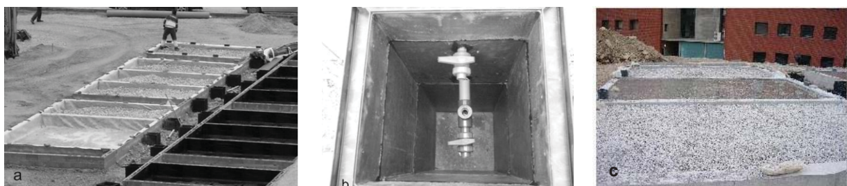
Figure 3: First steps of construction (a) watertight drawers with the sealing, (b) control manhole and (c) roadbed materials and sealing test.
