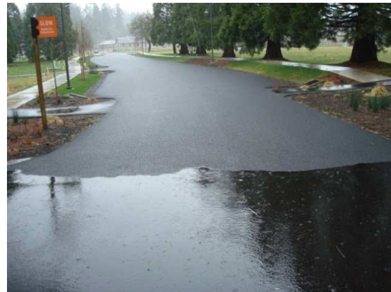
Figure 79: Permeable asphalt (The University of Rhode Island, 2005)
