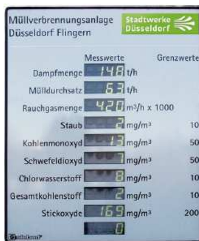
Figure 141: Digital display, viewable for the public outside of the plant (Stadtwerke Düsseldorf, 2010)
