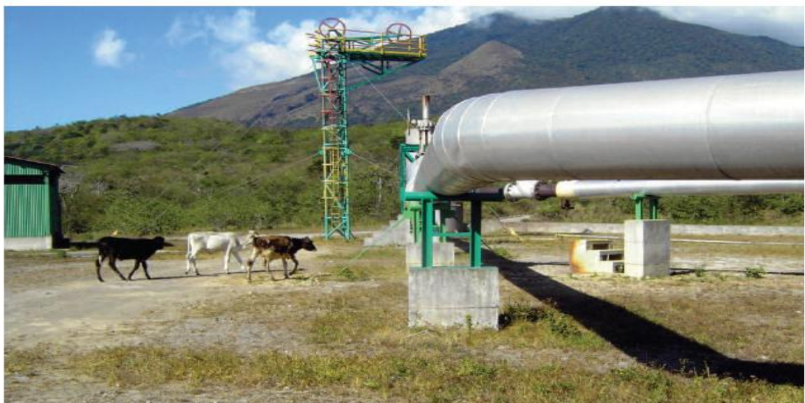
Fig E.5.17: Typical pipeline at Miravalles geothermal power plant, Costa (photo by R. DiPippo).
