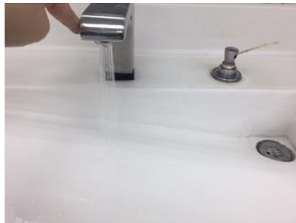
Image 4. Sink kind in the USFQ installations
