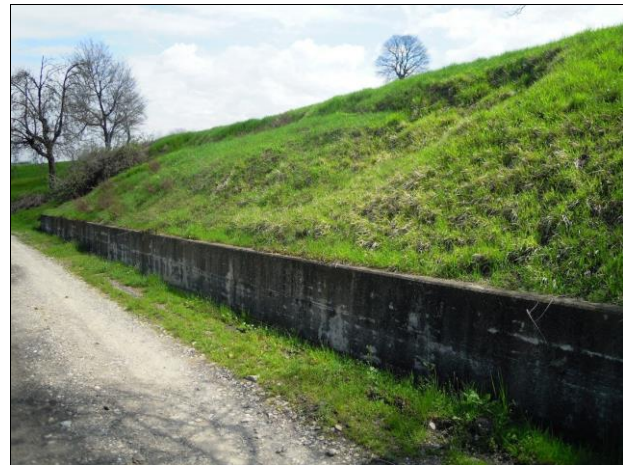
Figure 12 Upper Rio delle Vigne valley: eastern branch of the landslide which affected the road.
