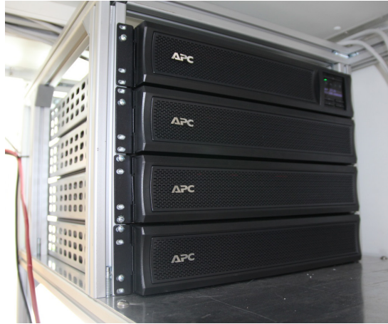
Figure 6: UPS mounted in the top compartment of the NDS rack
