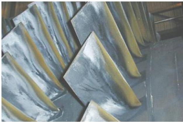
Figure 22: Low Solubility Deposits on Compressor Blades (Courtesy, Turbotect Ltd. )
