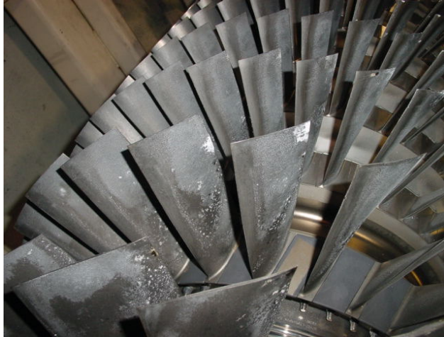
Figure 21: Salt Deposits on Compressor Blades (Courtesy, Turbotect Ltd. )
