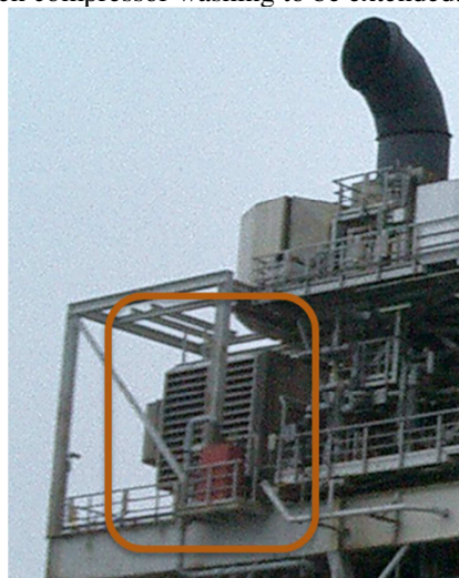
Figure 24:Traditional high velocity GT inlet system on board a north sea platform
