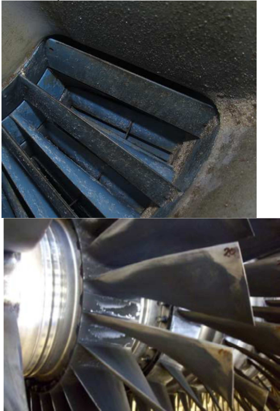
Figure 11: Compressor Fouling. Bottom Picture: Fouling due to Carbon Black Deposit.
