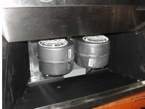
Figure 18: Range Hood Enclosure Modification (Code: ENC)
