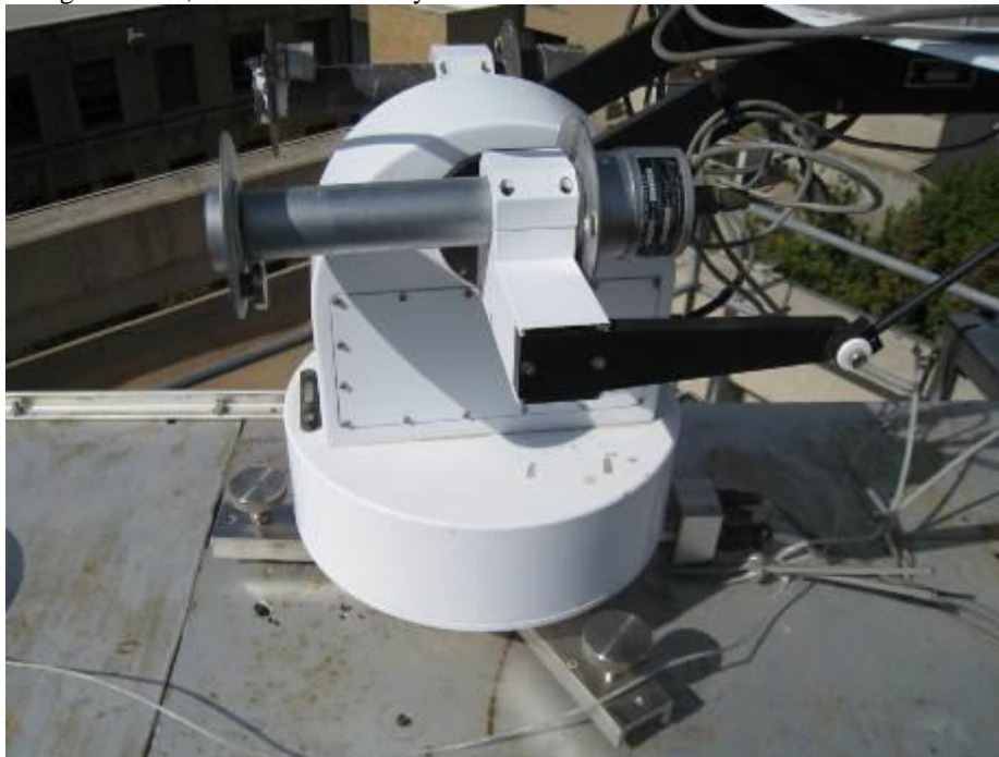
Figure 81. Solar tracker SMT-3 installed in the ESL Solar Test Bench
