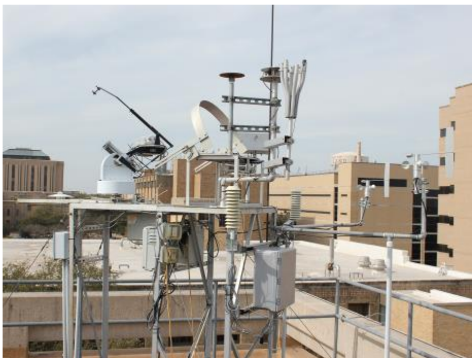
Figure 77. Solar Test Bench at the roof of Langford Architecture Center Building A
