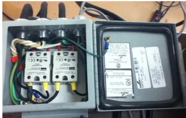
Fig 2.19–Solid state relays in electric box
