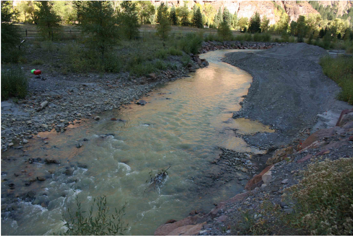
Fig. 34. R2 during late September 2010. The gravel bar has been prepared for excavation by bulldozing a large pile.
