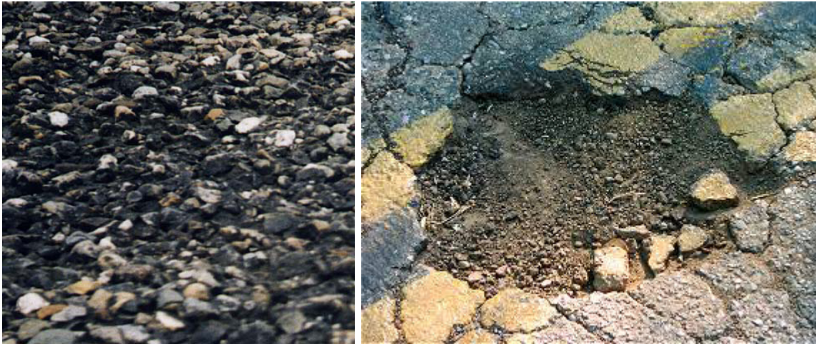
Figure 1.1 Moisture-induced damage in pavements results in raveling (left) and potholing (right) (Kringos 2007)
