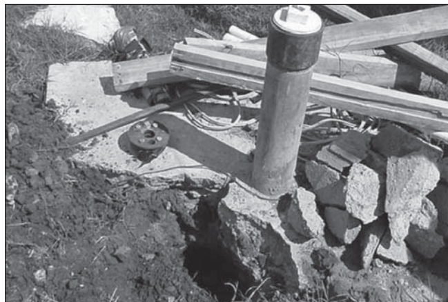
Figure 1. The slab around this capped well must be repaired to keep water from entering the well bore hole.
