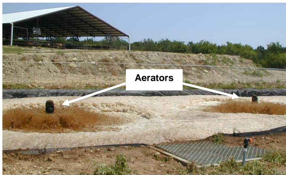
Fig. II.10. Aeration pool. (Broumley, 2005)
