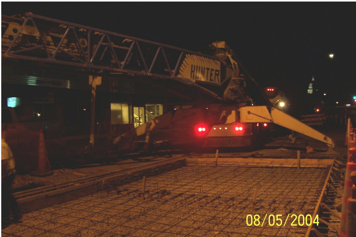
Fig. 6. Concrete paving at night at the intersection of 12th Street and Lamar Blvd.
