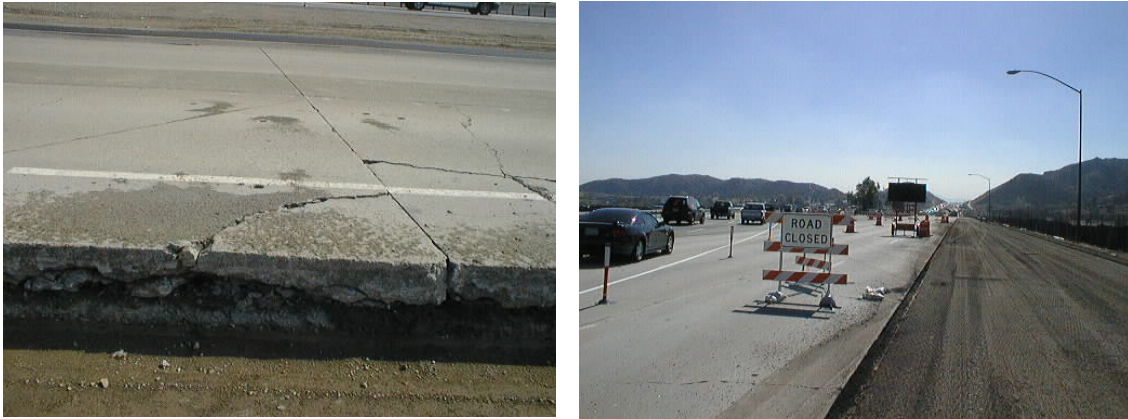
Fig. 10. Damaged concrete slabs in the outside lanes (left) and the beginning of construction workzone, southbound (right)
