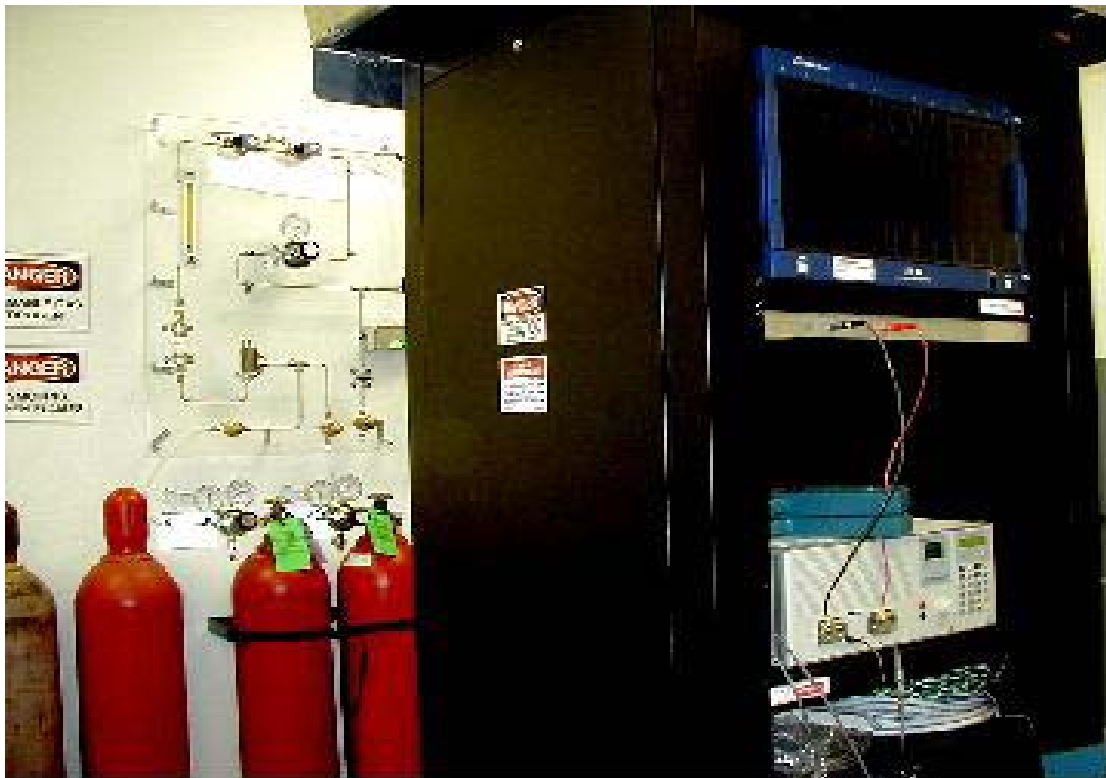
Fig. 3.6 Fuel cell system installed in the Power Electronics & Fuel Cell Power System Laboratory of Texas A&M University.
