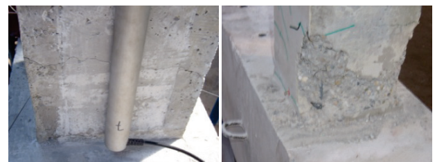
Figure 10 Crack patterns observed on the MODEL 10 columns
