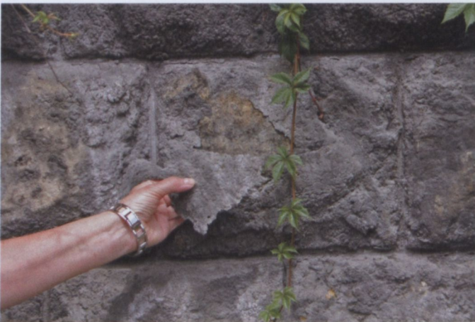
Fig. B15. Black crust on the wall surface subjected to dry and wet deposition (Kamienna Street, Kraków).
