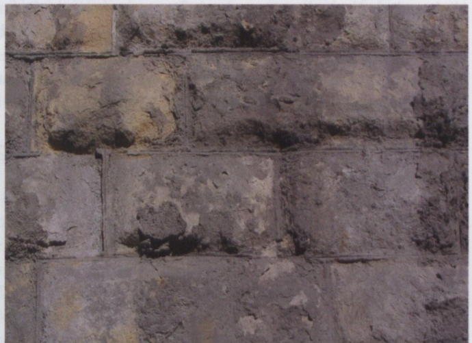
Fig. B22. Gypsum-rich crust on the surface of sandstone blocks (Lubicz Street, Kraków).
