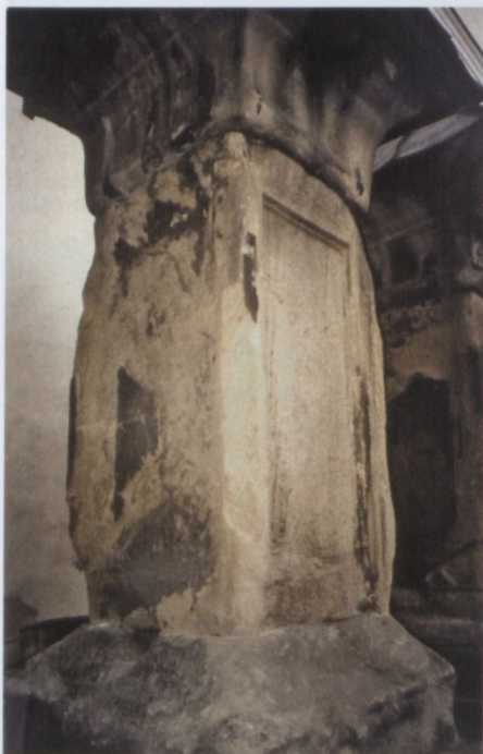
Fig. B23. Disintegration of sandstone block (St. Peter and Paul Church, Kraków).
