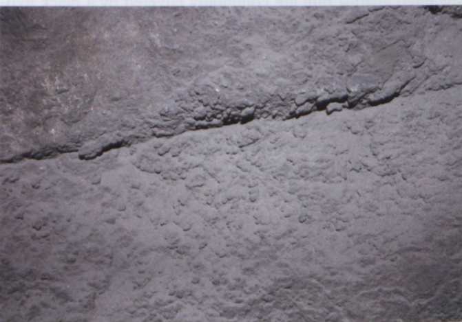
Fig. B16. Grey crust on the wall subjected to dry deposition (Łokietka Street, Kraków).
