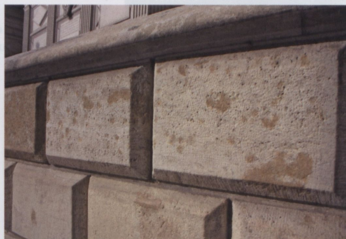
Fig. B13. Alveolae in the Libiąż dolomite, filled during renovation; wall around the Wawel Cathedral (Kraków).
