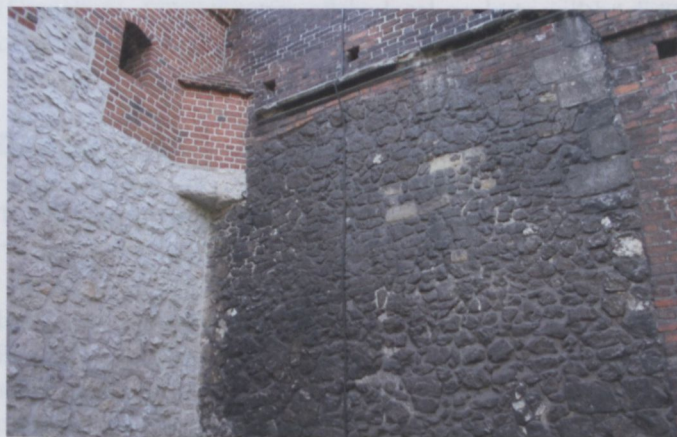
Fig. B1. City walls of Kraków before renovation (right) and after renovation (left).
