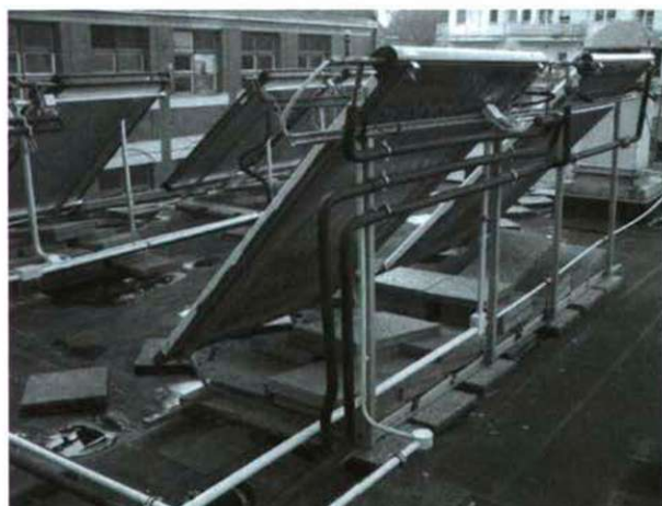
Figure 4. Measuring system with Buderus collectors
