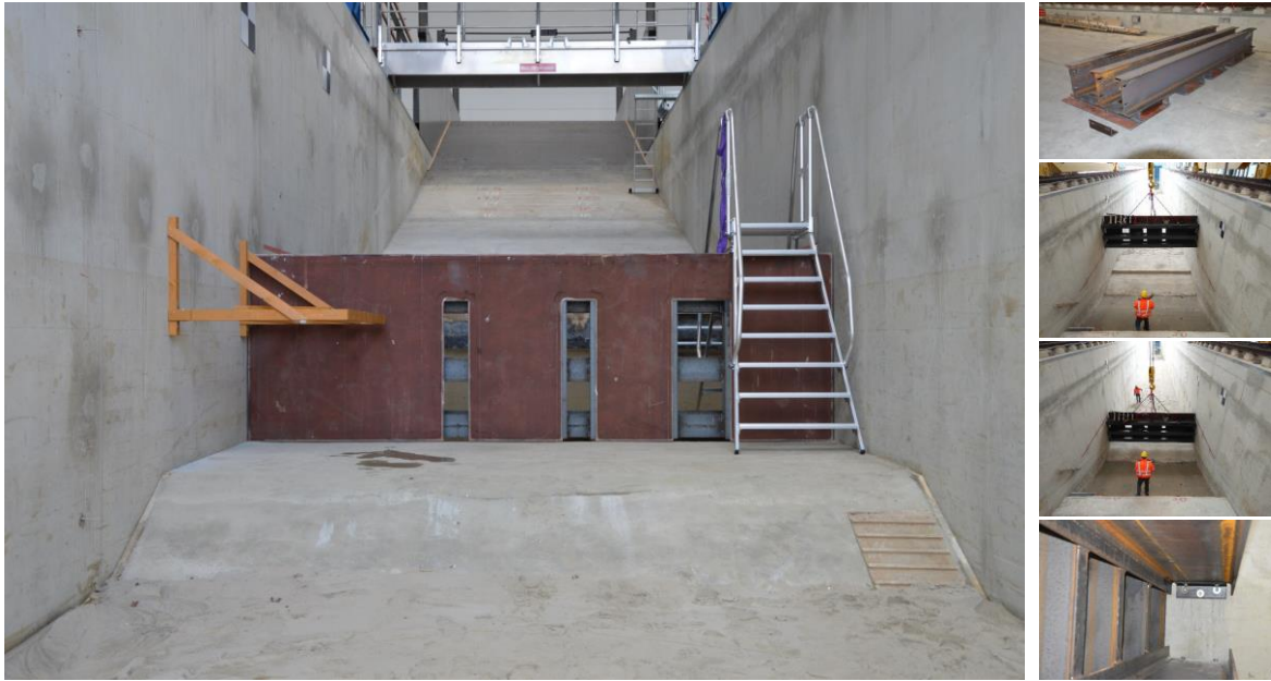
Figure 2. Steel wall as constructed in the Delta Flume with openings for the force and pressure measurement sections and an observation window. Images to the right show the installation of the steel wall.
