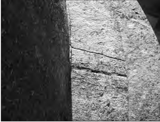
Fig. 3: Degradation of the dome
