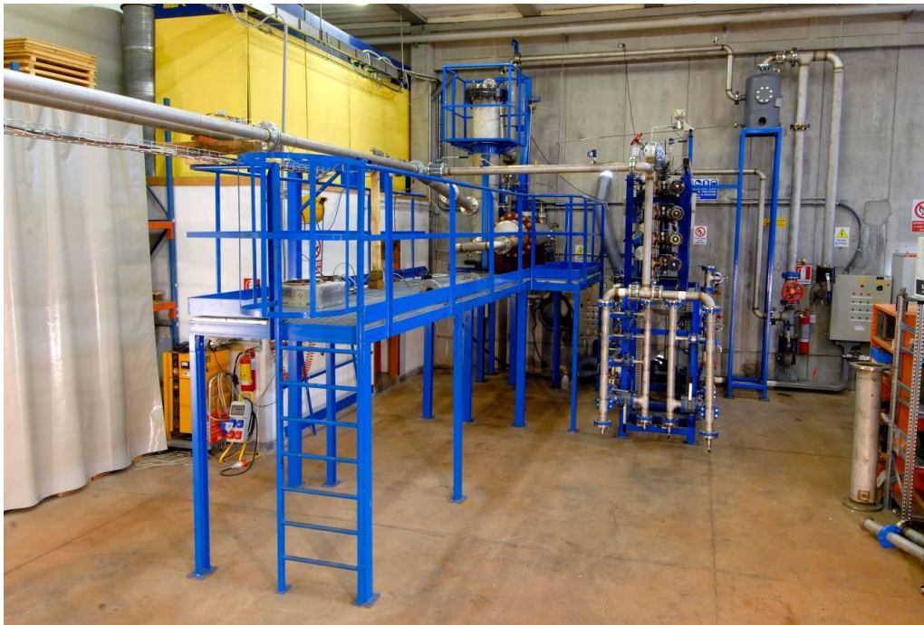
Figure 51: Panoramic view of the SESAME project facility
