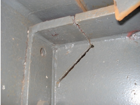
Figure 9: Typical fatigue damage and repair of track bracing cross beams
