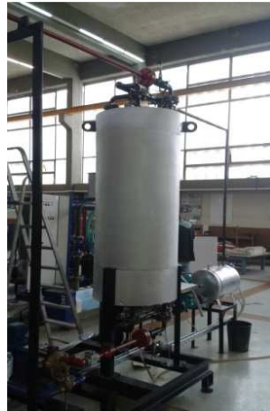
Figure 2. Helical coil heat exchanger installed in the laboratory in an ORC installation.
