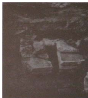
Figure 2.4 Mastic covered toilet seat
