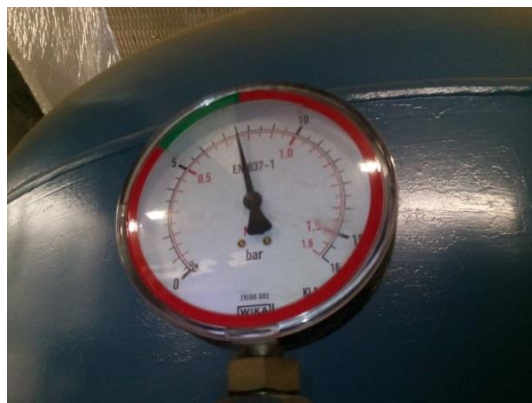
Figure 21: visual reminder on pressure gauge to facilitate checks
