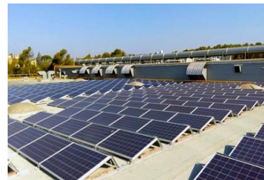
Figure 14: Rooftop PV at DENSO
