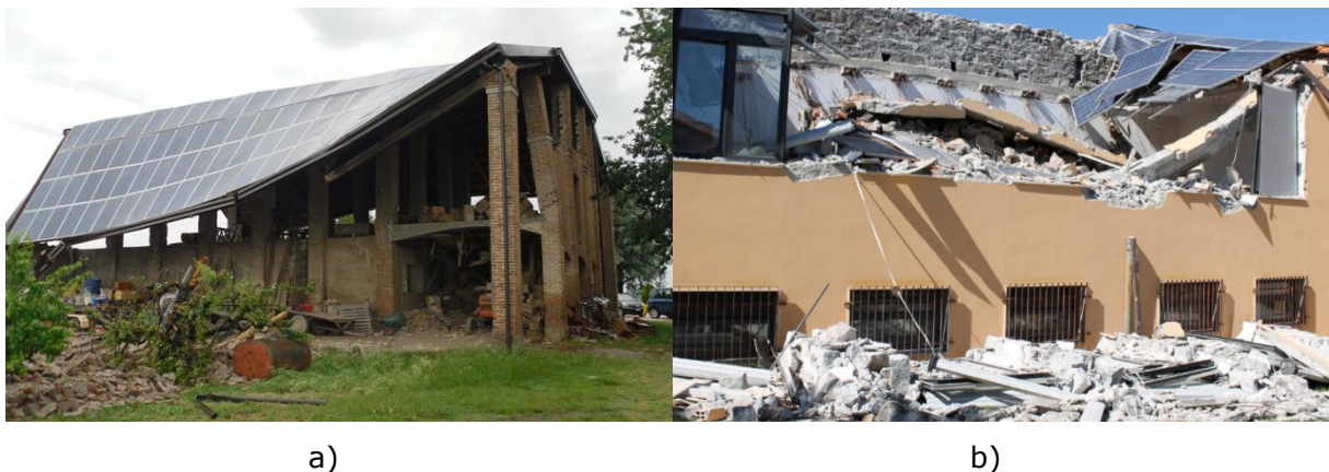
Figure 1. Examples of safety neglect in buildings with energy improvements. a) roof collapse of a building in Emilia Romagna Region (Italy) after the 2012 earthquake; b) roof collapse of a Municipal library in Sardinia Region (Italy) for gravity loads, in 2015
