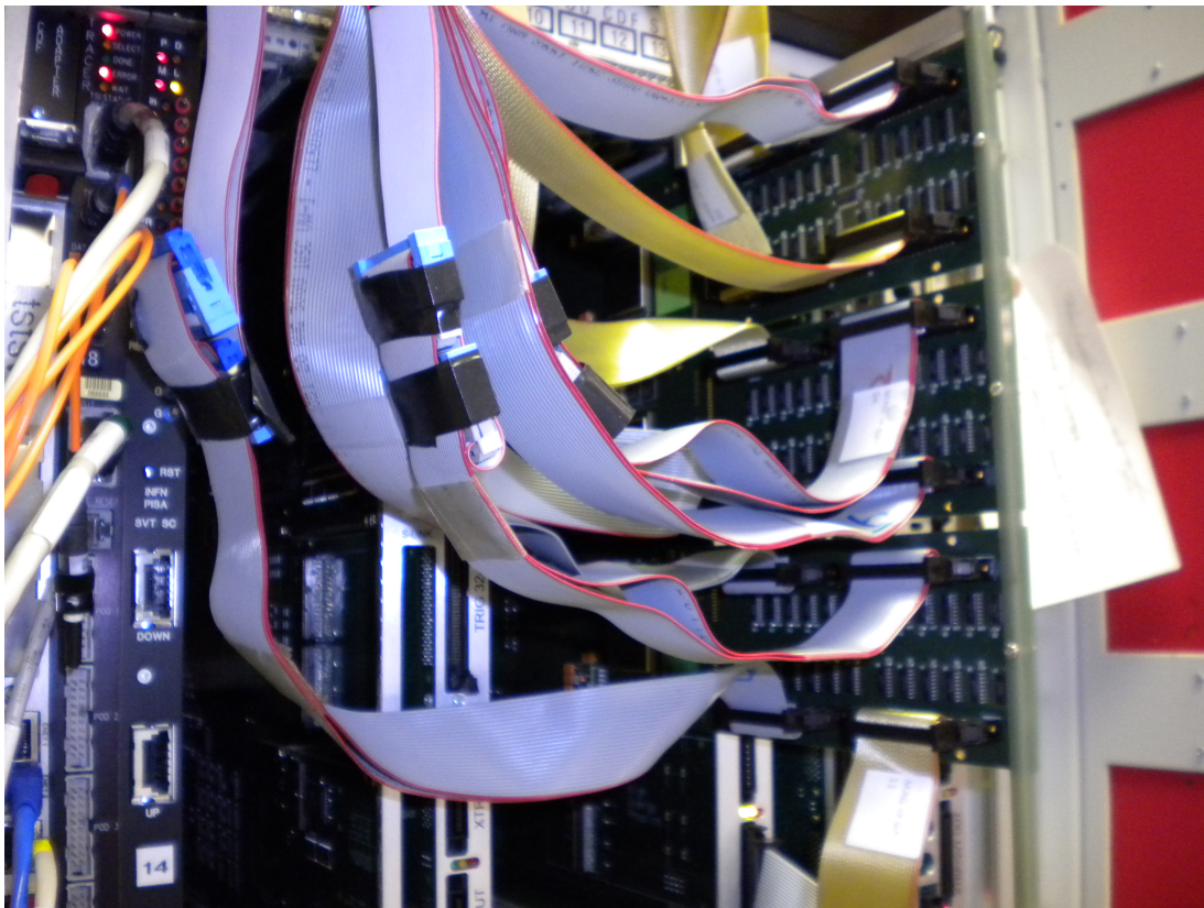
Figure 5.7: The GigaFitter system installed - The GigaFitter system in the test crate of SVT. All 12 input are connected in parasitic mode to splitted HB++ outputs.
