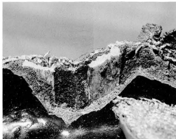
図74 刎足破損部の状態 Condition of damage of the kuriashi
