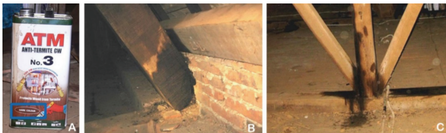
Figure 3. A) Insecticide used in the previous restoration intervention; B) treated end grain of an old rafter; C) sign of insecticide treatment on new beams of the roof.
