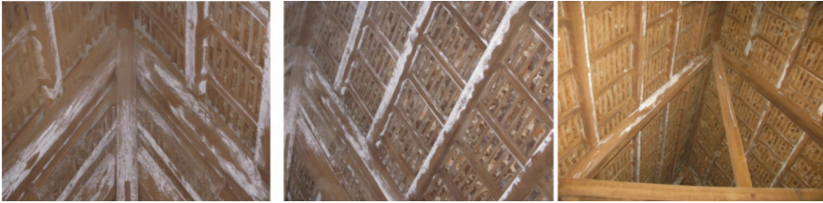
Figure 9. Detail of the fungi infestation found in the west wing of the Museum roof.
