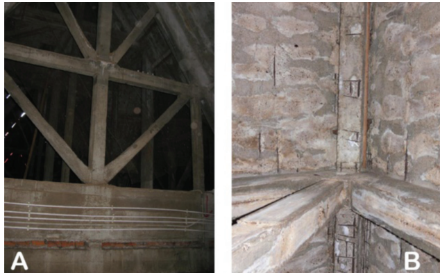
Figure 2. Concrete structure of the roof: A) base of the concrete structure with no visible corrosion of reinforcing steel bars; B) top of the structure with clear signs of corrosion.
