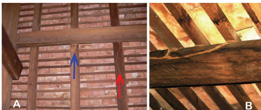
Figure 4. A) The blue arrow indicates a termite walkway on an old rafter, the red one indicates ghost traces of the walkway removed during the previous intervention; B) termite walkways on newly installed rafter.
