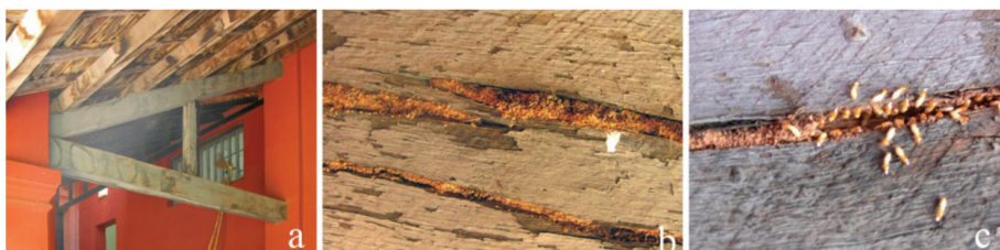
Figure 7. Colonnade beam: a) fungi signs; b) termite pathways; c) living termites.
