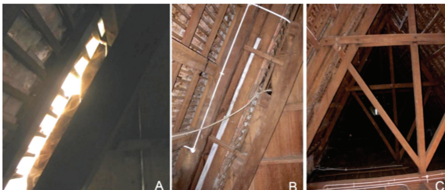
Figure 10. Roof structure: A) open gap between the folds of the roof; B) open gap between the folds sealed with tape; C) open gap between the folds sealed with mortar.
