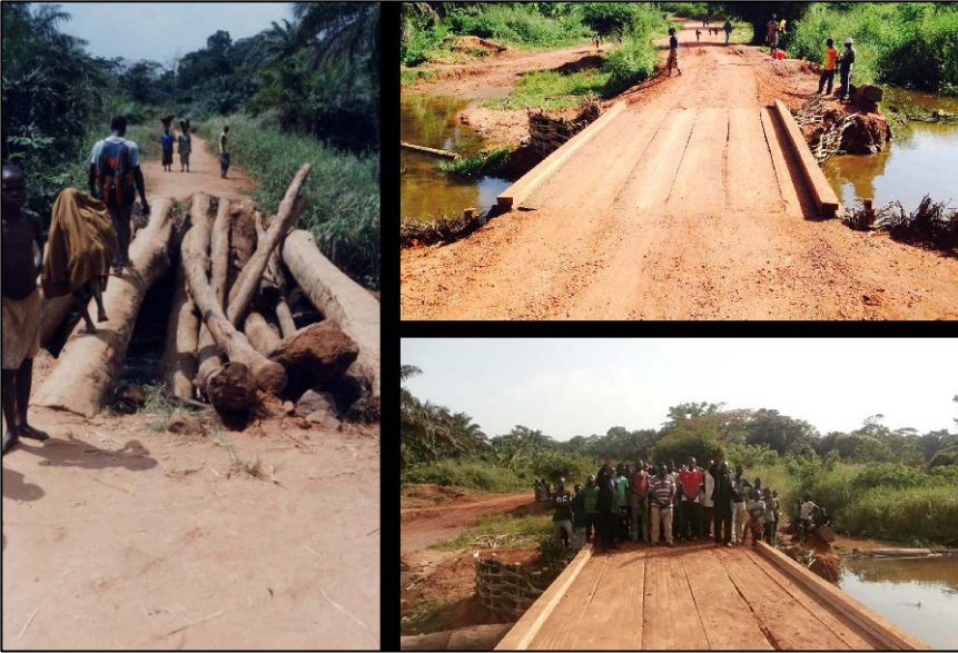
A bridge on the main road between Karawa and Loko in 2005 (on left), and another bridge on the same road that has been repaired by a local engineer and his team, with support from the Paul Carlson Partnership.
