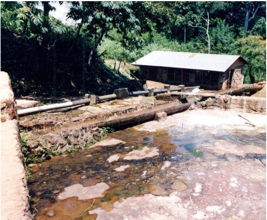
A microhydro mill in the Ubangi Subregion. The dam at the left edge of the photo diverts river water through a penstock to the turbine house, where it powers a small (six-twelve inches in diameter), locally made turbine.
