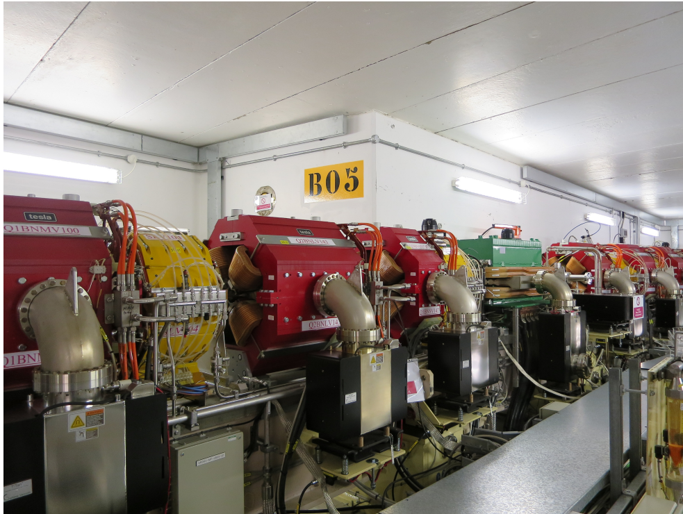
Figure 1.3: Inside Diamond Storage Ring tunnel showing quadrupole (red) magnets, sextupole (yellow) magnets, dipole bending (green) magnet, the vacuum ion pumps and the ratchet wall.
