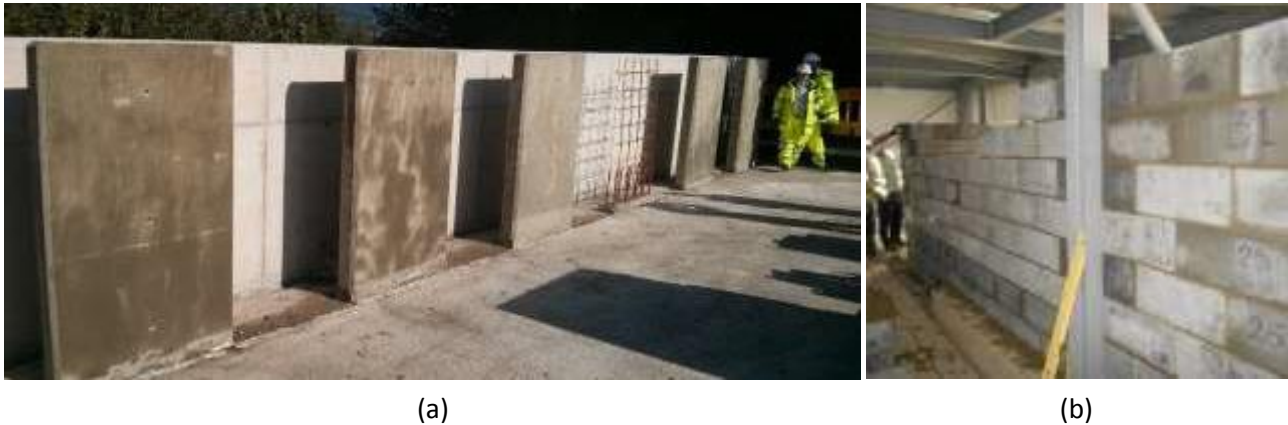
Fig. 5. Demonstration and commercial application of self-healing concrete in 2015: (a) Field trial panels on the A465 site and (b) concrete blocks in the new James Dyson Building in Cambridge.
